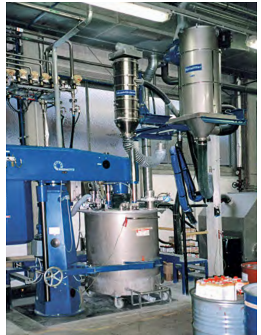
Vacuum conveyor for conveying pigments in the manufacturing of paint.
