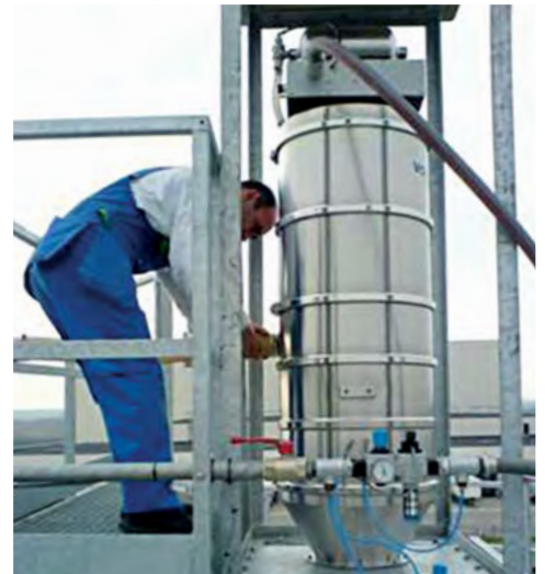
Vacuum conveyors in an outdoor installation, for charging silos.
